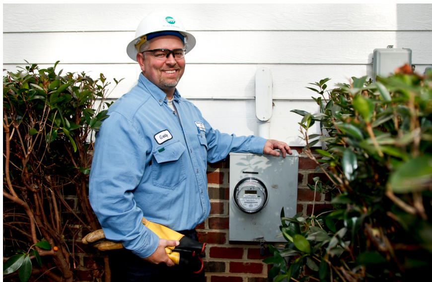
Wake Electric meter technician Grady Perry proudly installs a new AMI meter at a member's home.
