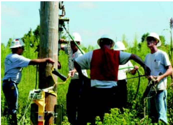
Wake Electric employees Tony Kearney, Chris Baker and Clark Blackburn install a variety of equipment used to raise a transmission pole down at the Emit Substation. Work was done with 69,000 volts pulsing in the lines overhead.
