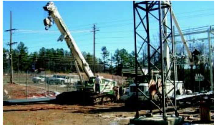
Providing reliable electric service is still the primary mission of Wake Electric. A new substation started during 2004 will improve service to members in its area.
