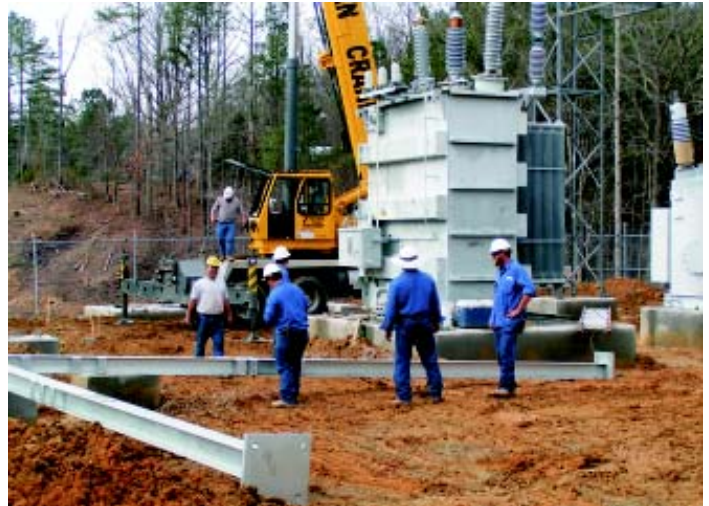
Work is underway at a new substation near Kittrell. A crane was used to lift a transformer in place.
