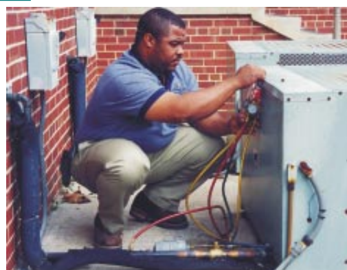
Wake's subsidiary, Triangle Services Group, Inc., offers a variety of services, including HVAC installation, service and repair.
