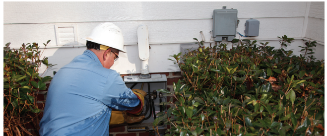
Wake Electric meter technician Grady Perry installs an AMI meter at the home of Wake Electric member.
